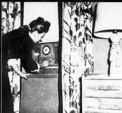
Addition of an automatic timer will permit the ventilator to go on for any length of time within a 12-hour period. The wiring diagram is on the next page.
